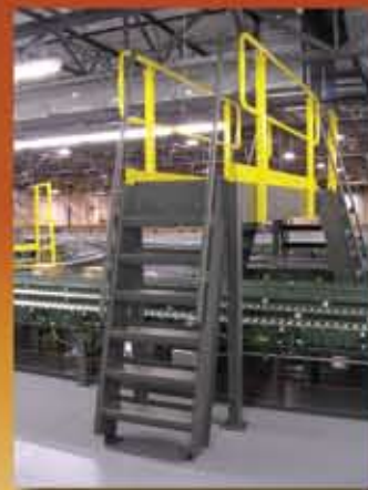
Custom-designed crossovers with ship's ladders and railings allow workers to safely access production areas without stopping workflow.
