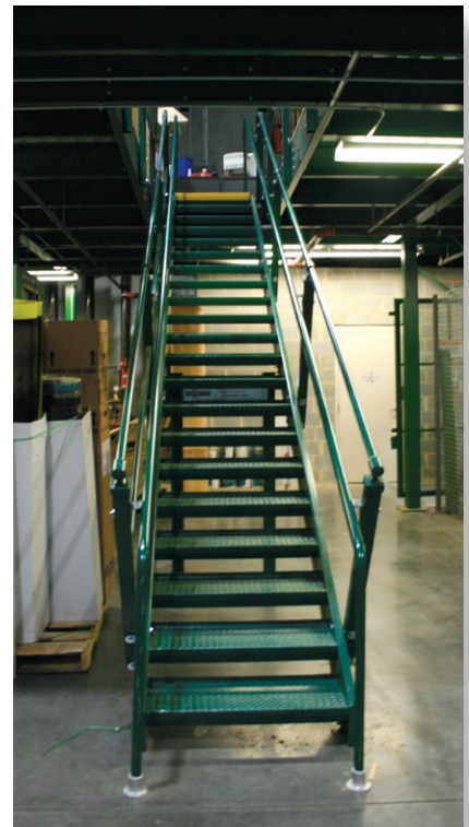
Fully welded Wildeck® stairs provide safe access to the mezzanine level at multiple locations.
